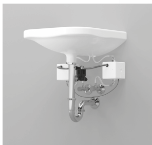
Installation as single device or warm/cold combination
